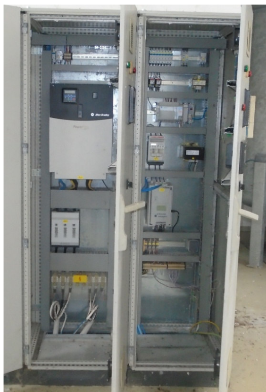
Automatika pumpe br. 4 i muljne pumpe
